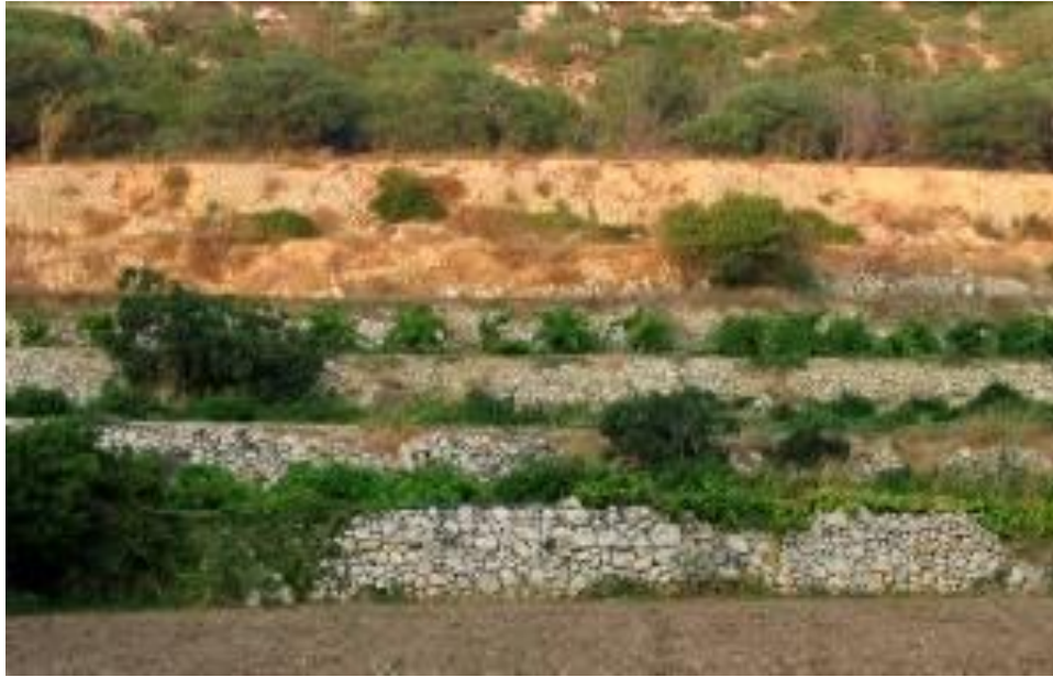
Fig.16: Soil slumps are observed in the upper terrace. Lower terraces show better maintained rubble walls (Wied Għemieri, Malta).
